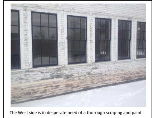
The West side is in desperate need of a thorough scraping and paint
