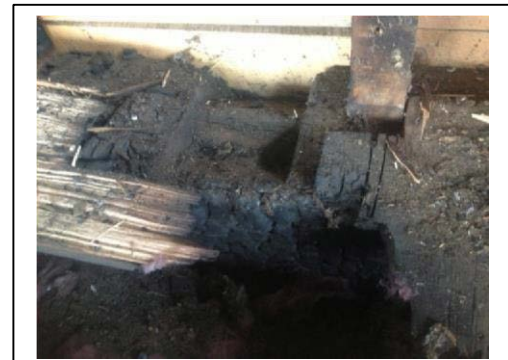
The charred horizontal timber is the original top plate to the building, now at the second floor level. The notch in the center of the beam is a step lap pocket, in which, the rafter once sat
